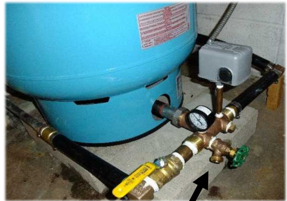
Pressure tank sampling tap
